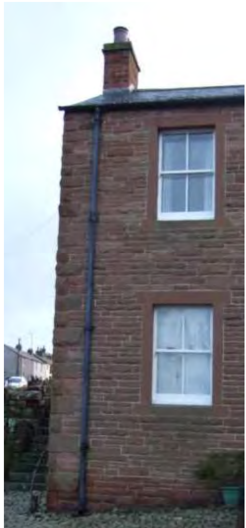
Figure 15 Typical decorative style from the village with emphasised quoins at the wall corner, simple junction with the eaves and flush fitting sandstone window surrounds. The walls are rough-dressed sandstone ashlars
