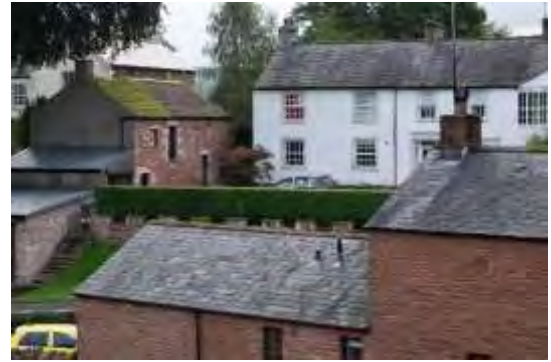
Figure 29 A variety of roofs: slate in foreground and background, with sandstone slabs on building to left with modern profile sheeting on lean-to
