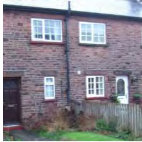
Figure 23 Fairly modern houses with side-hung casements. The windows have a sandstone lintel above, a sandstone sill and undressed sides. The windows are mix of top- and side-hung casements
